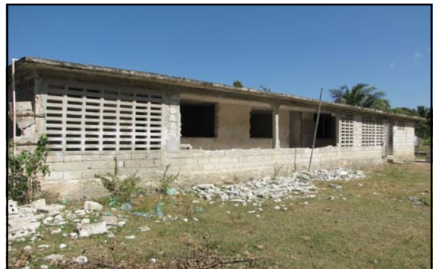
Although the school was damaged, with some repairs it will be useable again.
