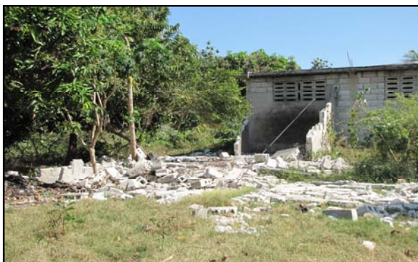
The school hot lunch program kitchen after the earthquake.
